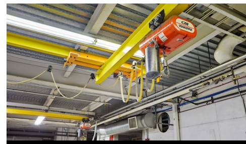
Building 1 - Bridge Crane
